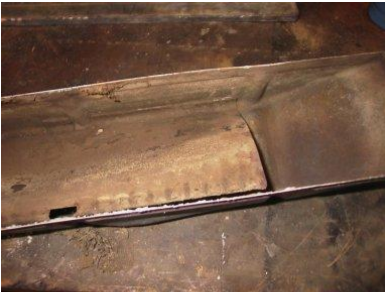
13. Baffle was loose in most parts:
